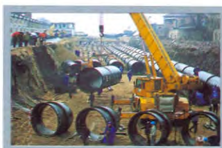
新兴铸管用于武汉排渍工程 Xinxing pipes are used for rain water drainage project in Wuhan, China
