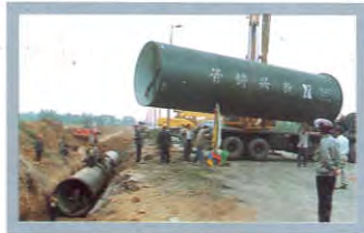
大口径新兴铸管首次成功用于太原引黄工程 Large diameter pipes are successfully used for Yellow River Diversion Project in Taiyuan
